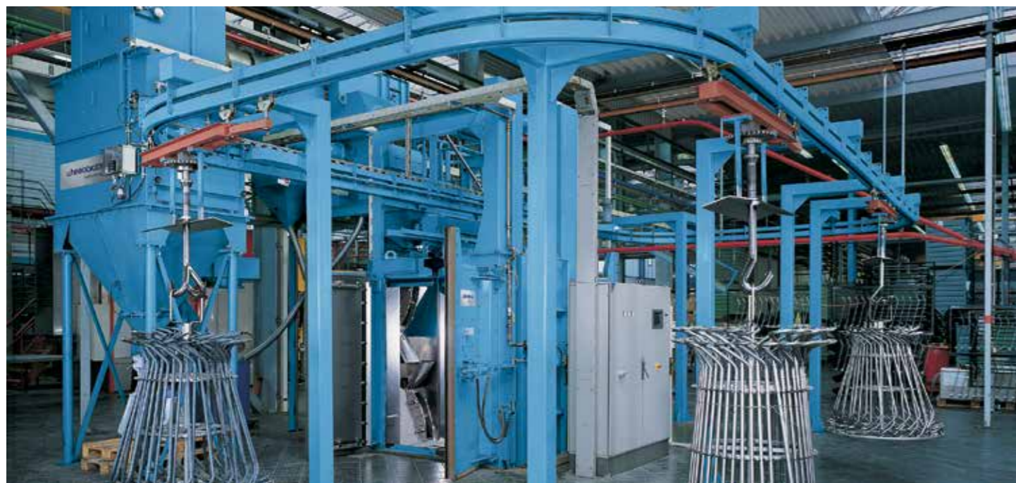
Hanger type solution with monorail for shot peening of stabilizers
